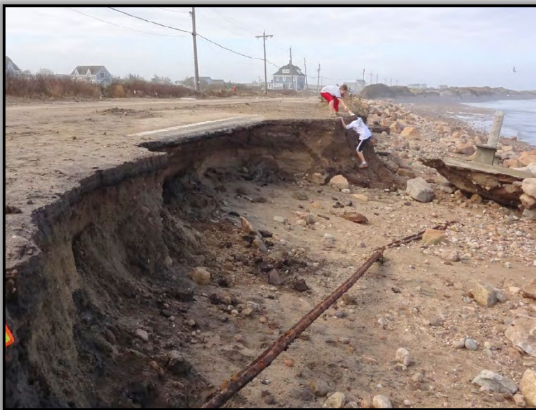
Damage to Corn Neck Road from Superstorm Sandy (2012)
