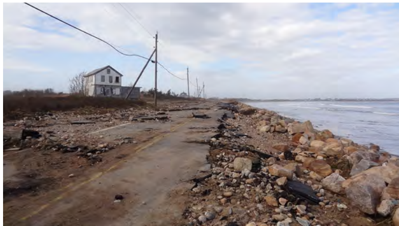
Corn Neck Road in the aftermath of Superstorm Sandy
