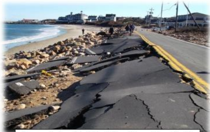
Damage to Corn Neck Road from Super Storm Sandy October 2012
